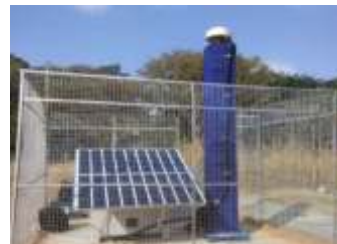
CORS Station Setup
